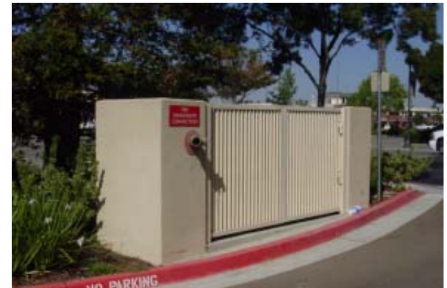
Backflow preventor is screened by wall and landscaping.
